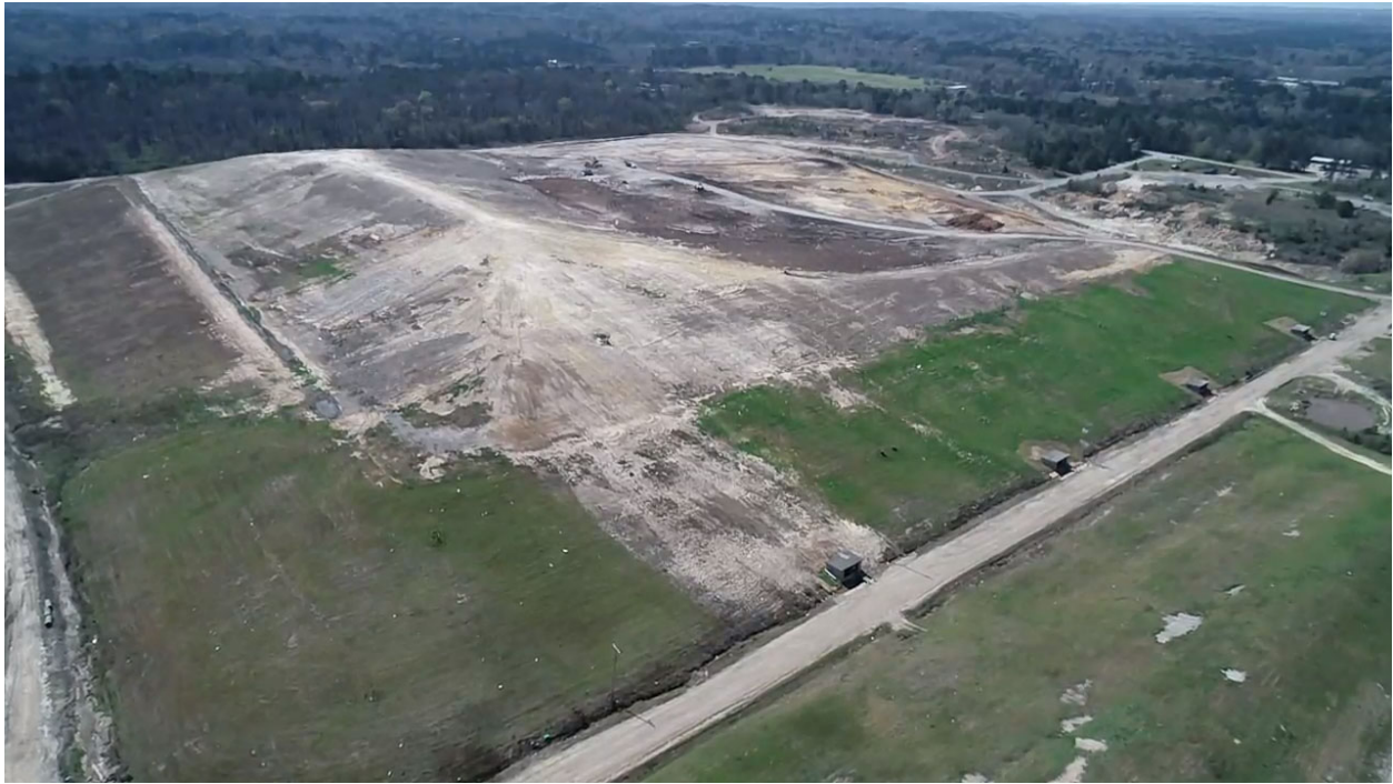
Looking SW over north slope of Cells 1 and 2 – active area in background
