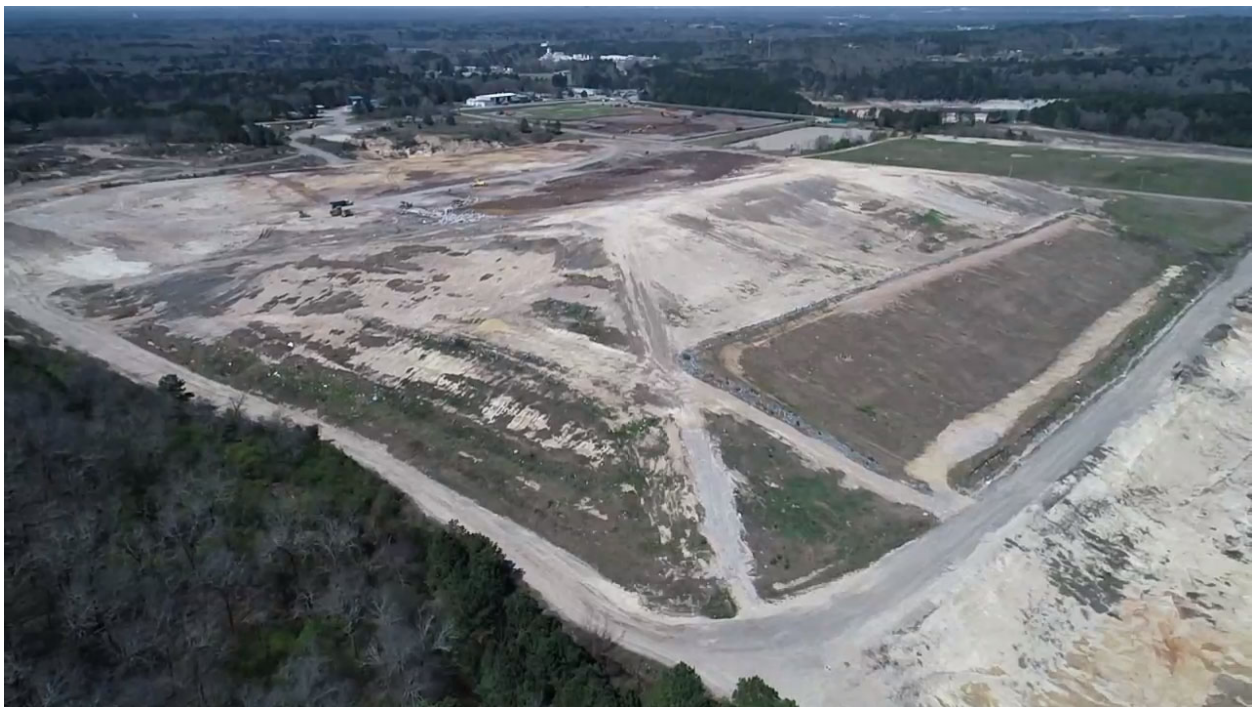
Looking NW over east slope of Cell 4 – partial closed area on the right
