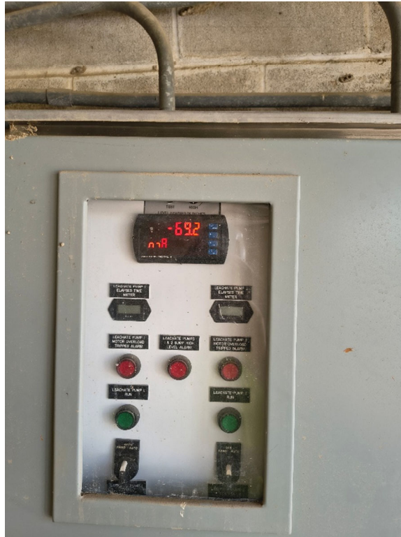
Documenting leachate level controllers
